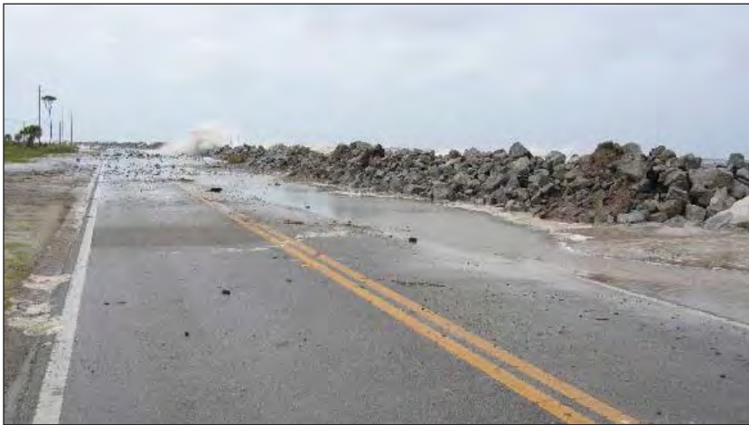
Figure 6-2B. Highway 30E at Stump Hole on the St. Joseph Peninsula during a storm event.
