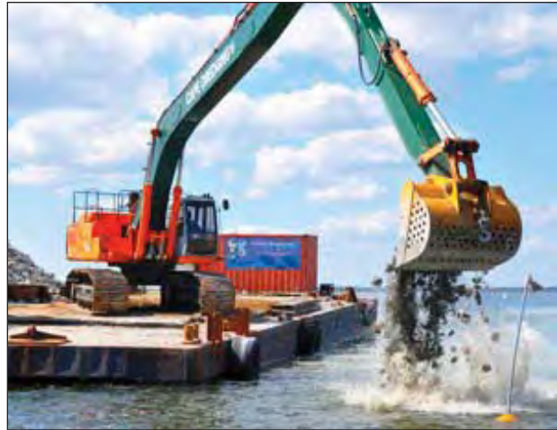
Figure 7-2C. Cultch being placed on a bay bottom from a barge for restoration (source: White 2012).
