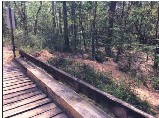
Figure 3-4D. Dorcas Road at Pond Creek Bridge with significant sedimentation next to the bridge.
